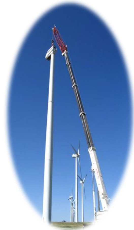
Test Turbine at Ponnequin/Photo by Jeroen van Dam, NREL 19257
